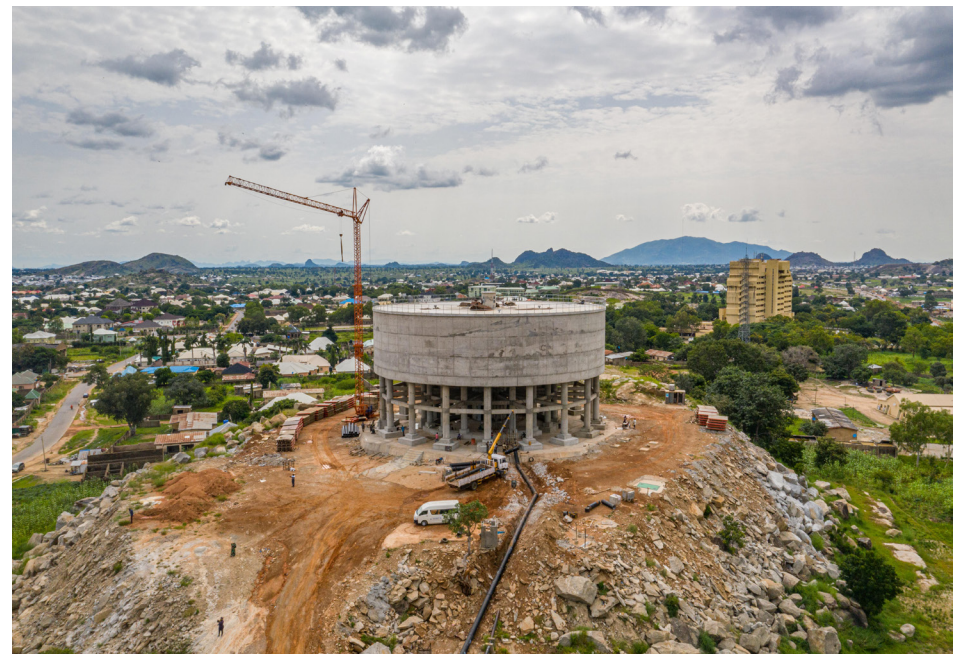
7000 cubic metres reservoir in Buzaya, Bauchi State
