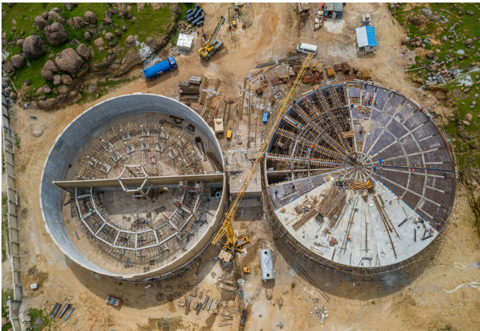
Twin 11000 cubic metres reservoir in Waringe, Bauchi State
